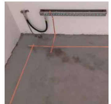
Copper strip, connected to earth bar.
