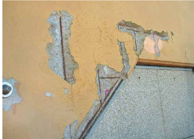
Spalling on a facade due to inadequate concrete cover.
