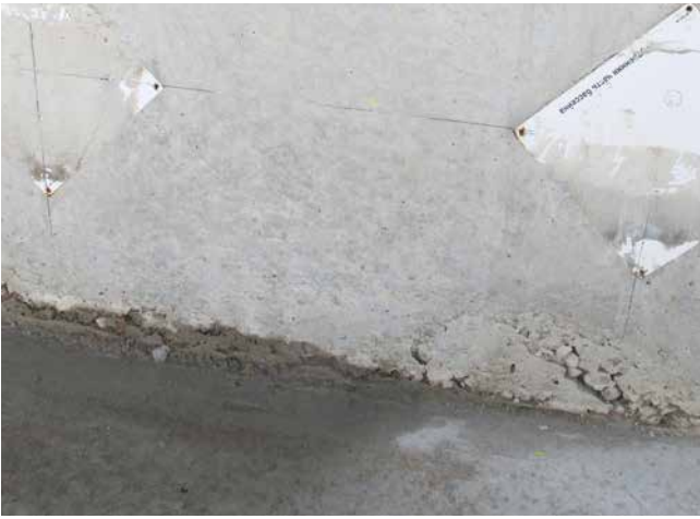
Honeycombing at wall/floor junction.
