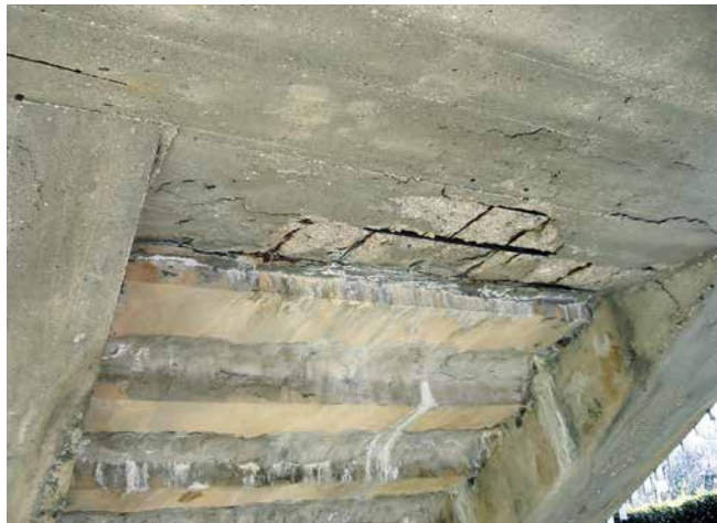
Corrosion damage to a stair soffit caused by lack of waterproofing and inadequate concrete cover.
