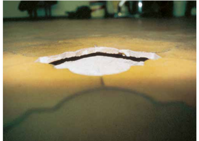
Voids in tile bed.
