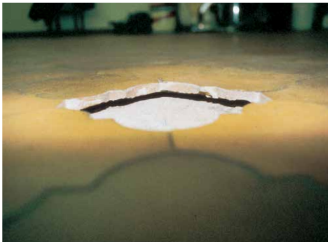
Voids in tile bed.
