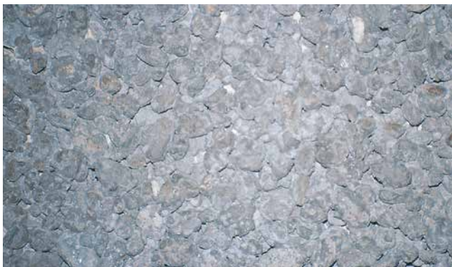
Porous cement screed.
