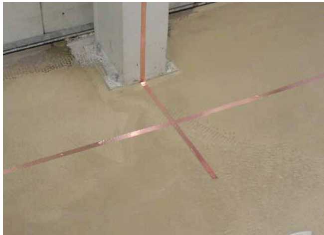
4 Copper strip laid on vertical element for later connection to equipotential bonding system.
