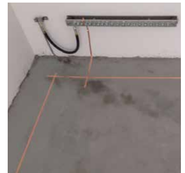
Copper strip, connected to earth bar.
